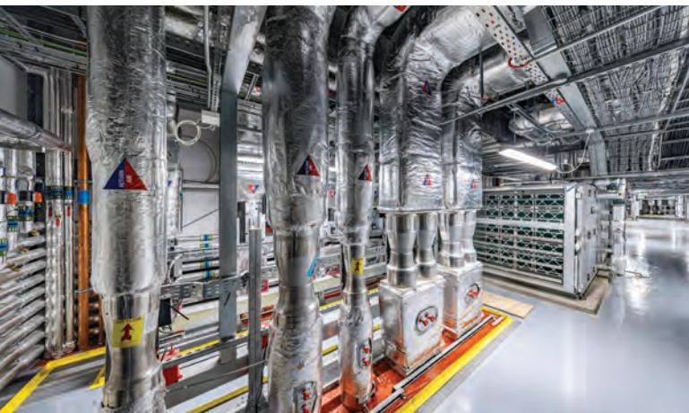
Ductwork servicing critical laboratory extract systems utilising venturi valves
