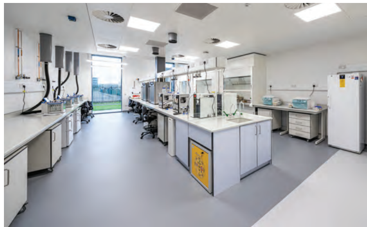
Interior of one of the water testing laboratories featuring mechanical ventilation system
